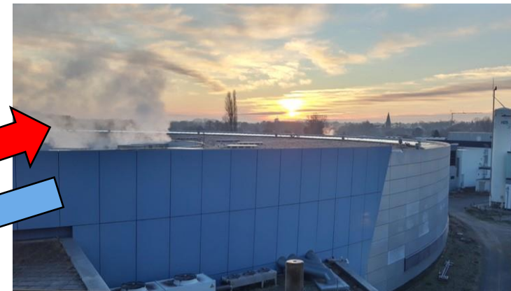
Evaporating cooling system
