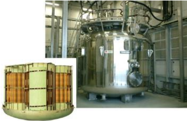
SMES: 10 MVA 10 MJ, 6.6kV, 1400A
