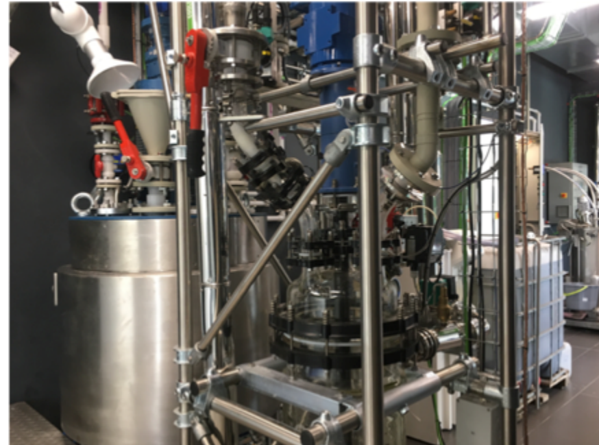
GO Pilot plant
